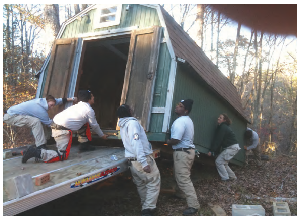
AmeriCorps team members moved this barn to create a larger playfield in the youth camp area. The barn, which has gone from being a Garden Shed to the Archery Storage Shed, will be reused as the Waterfront Barn for life jackets and paddles shed!
